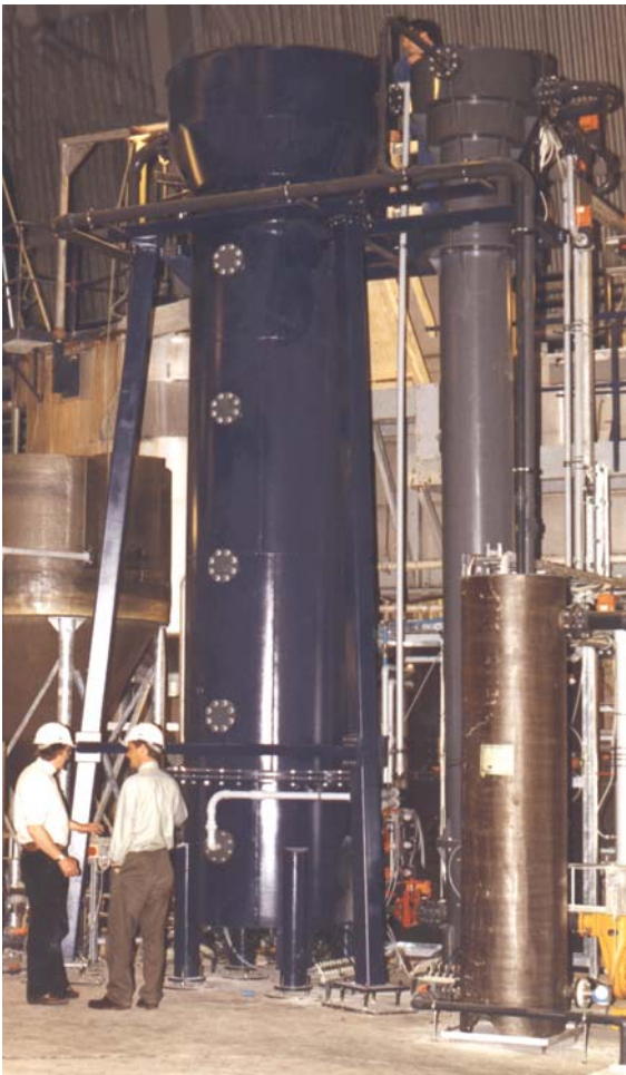
A 30 m 3 /hr reactor under construction at Avedøre, Power Plant, Copenhagen - Danmark
