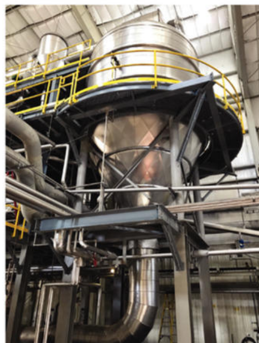
1. A forced-circulation HPD crystallizer integrated into Veolia's CoLD process (crystallization of high-solubility salts at low temperature and deep vacuum) is shown here during commissioning at a steam-electric site in 2019. Courtesy: Veolia Water Technologies
