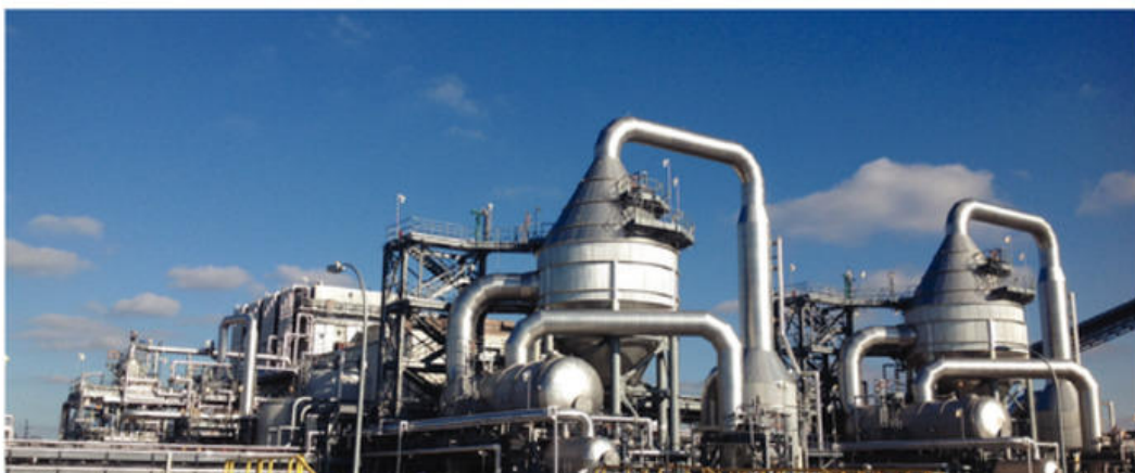
2. The CoLD process is founded on HPD evaporation and crystallization technology—a water treatment solution Veolia has been using for more than 85 years. Courtesy: Veolia Water Technologies
