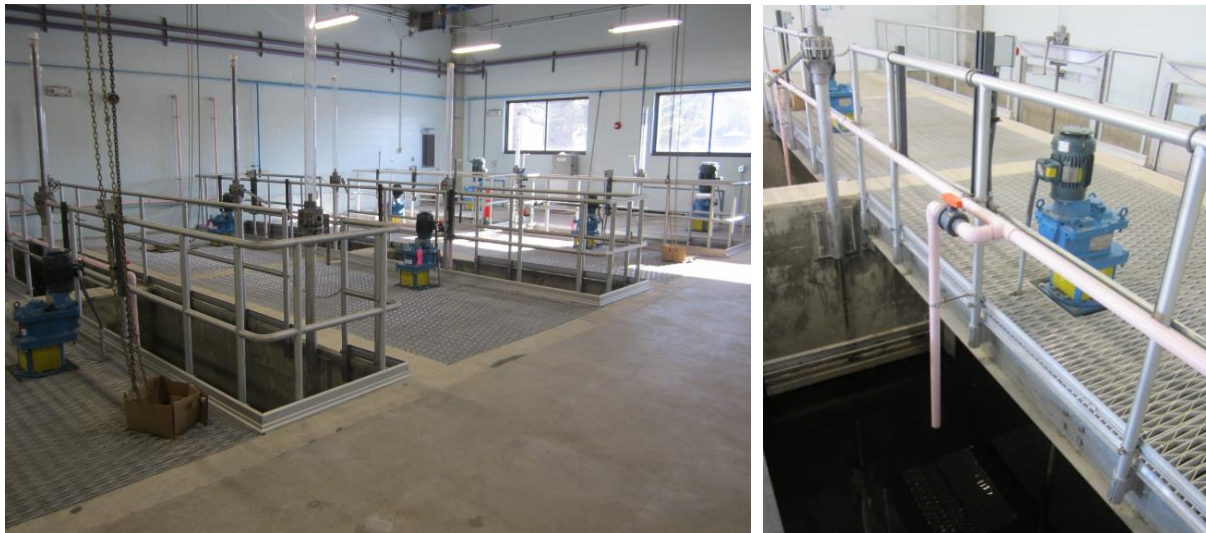
Figures 3 & 4: Mixing Zones with Chemical Dosing Upstream of Discfilters
