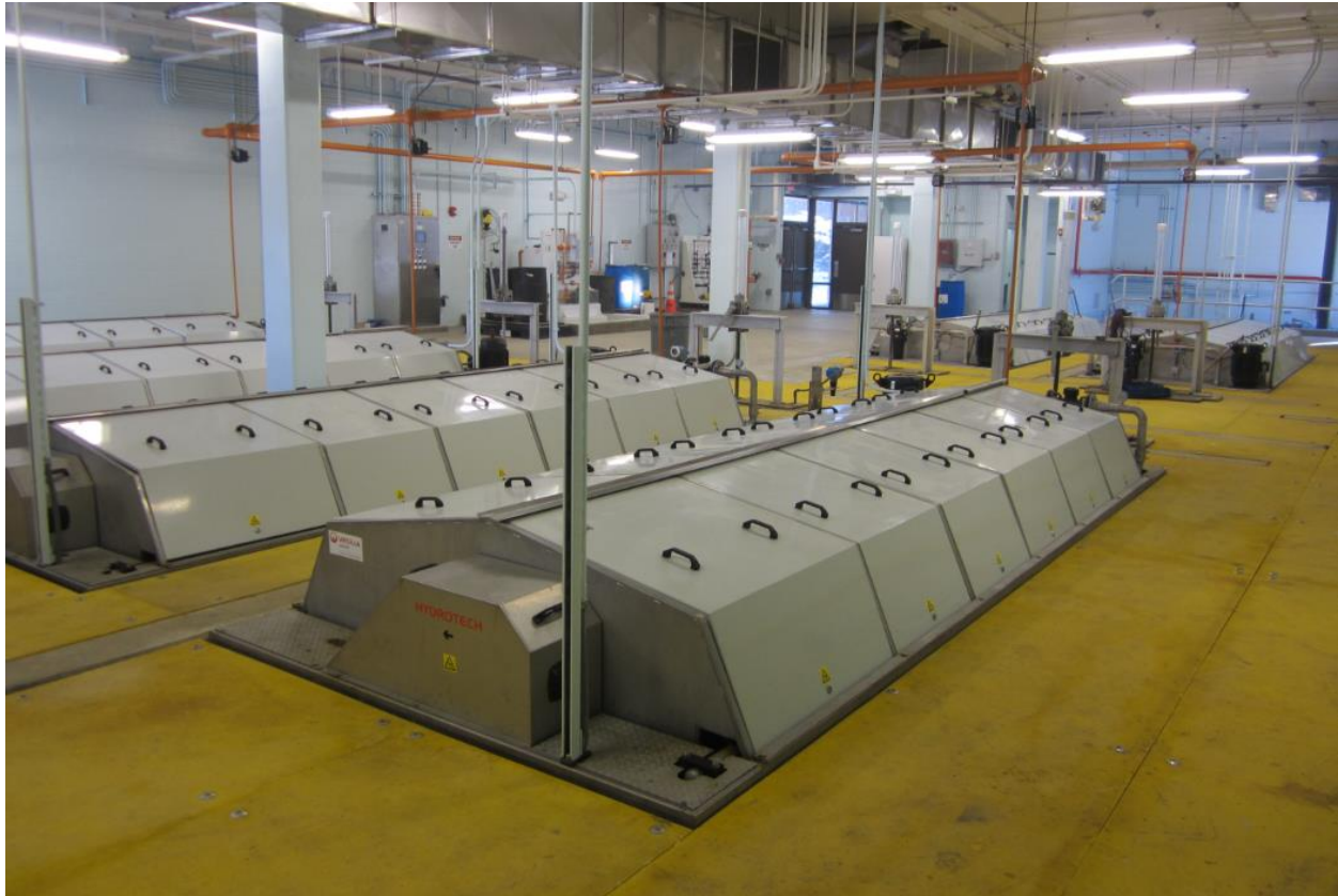
Figure 5: Hydrotech Discfilter Units Installed in Existing Filter Building
